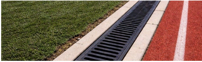
300 linear feet of Swift Drain 6" pre-sloped trench drain — ADA-compliant grates flush with track surface, Tennessee, 2021
